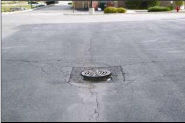
Defect 1: This catch basin is higher than the surrounding asphalt.
