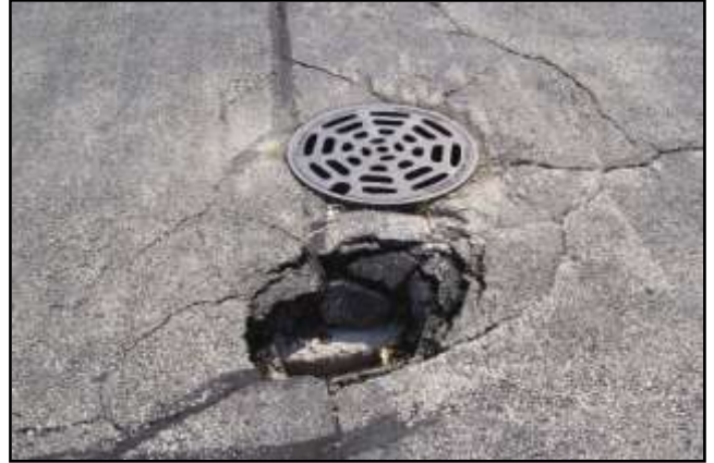
Defect 2: A sinkhole has developed adjacent to the catch basin.
