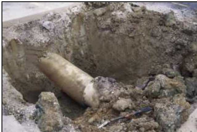
Defect 3: A collapsed pipe.
